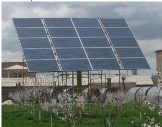
Fig. 3. Demonstration PV station
